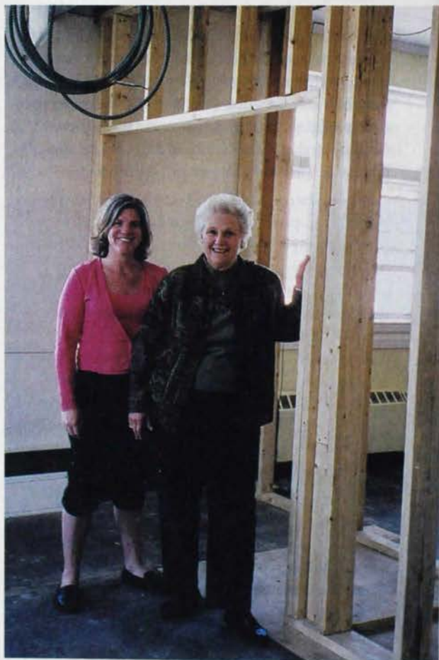
ROSALYN KEMPTON WOOD, Emory , and Esperanza Academy Head of School Laurie Bottiger inspect building renovations.
